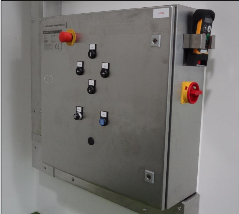
Controls mounted on a switchboard cabinet.
